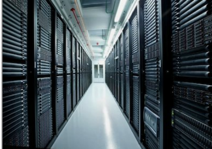
Cloud Data Center
